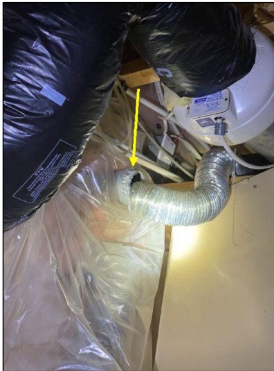
Damaged vent pipe noted.
