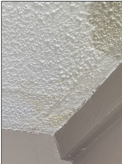
Small stains noted on the basement ceiling. They tested dry at the time of the inspection.
