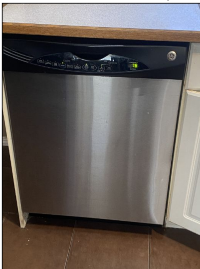
Operated. Functional. It was in good operational condition at the time of inspection.
