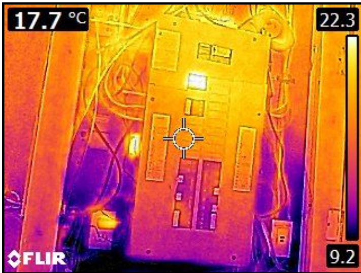
No major system safety or function concerns noted at time of inspection at main panel box.
