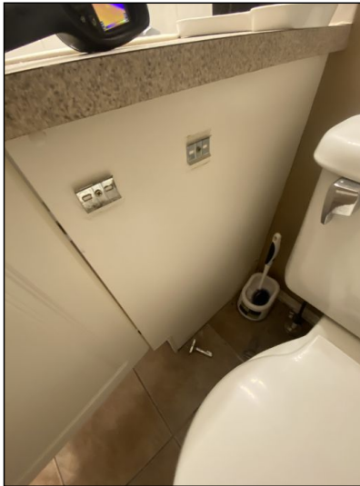
Missing toilet paper holder.
