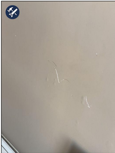
Some damaged walls noted throughout the house.
