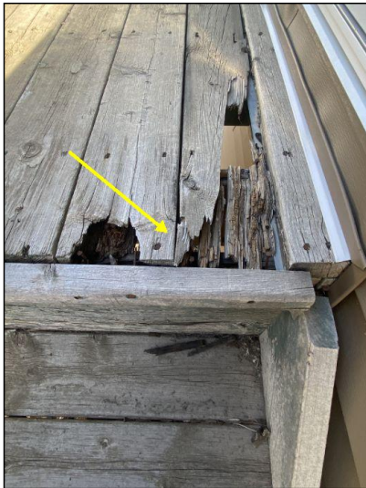
Front and side deck Floor boards rotted. Recommend repair by qualified contractor.
