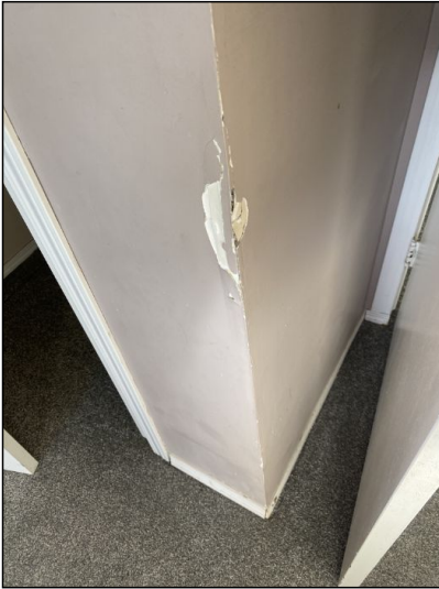
Some damaged walls noted throughout the house.
