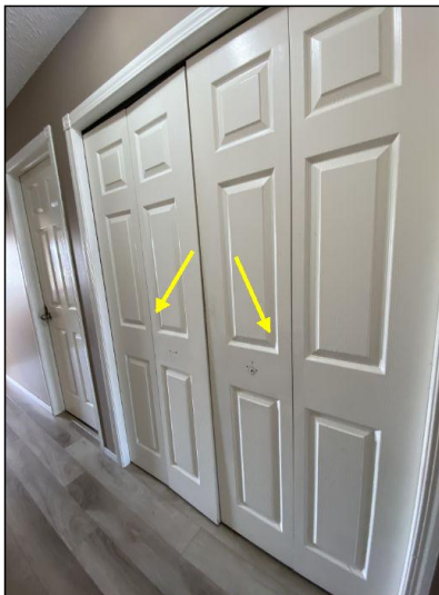
The closet doors handle/knobs are missing.
