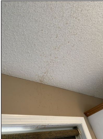
Small stains noted on the ceiling. They tested dry at the time of the inspection.
