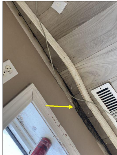
Mold like stains are present under the baseboard. We recommend further evaluation by qualified contractor.
