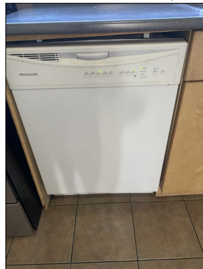
Operated. Functional. It was in good operational condition at the time of inspection.
