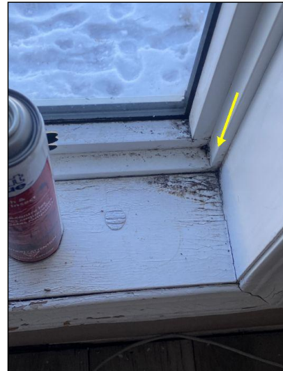
One or more window/s shows sign of loss of seal/condensation, evidence of past leak observed recommend repair or replace to provide energy savings and prevent hazed window from limiting view out of window.
