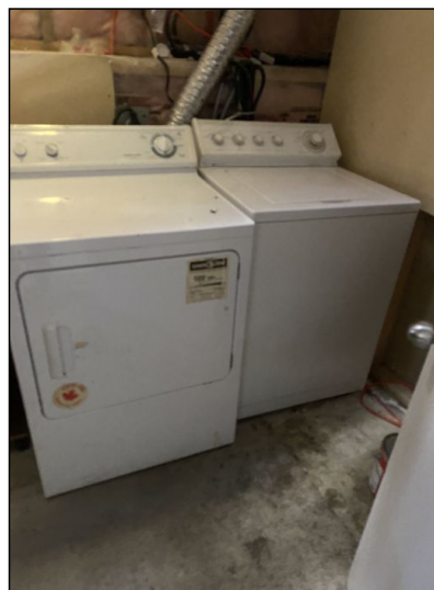
Laundry appliances were operational at the time of inspection.
