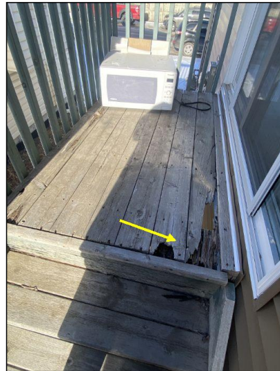
Front and side deck Floor boards rotted. Recommend repair by qualified contractor.
