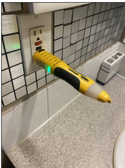
GFCI in place and operational
