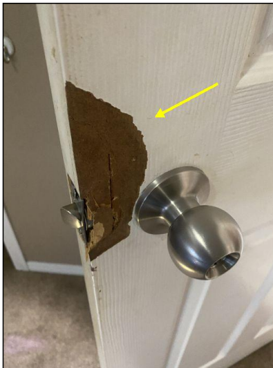
Some doors are damaged.
