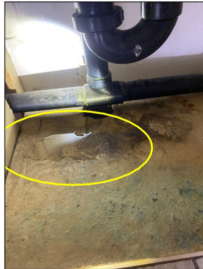
Visible leaking noted under the sink. We recommend contacting a licensed plumbing contractor for repair options.
