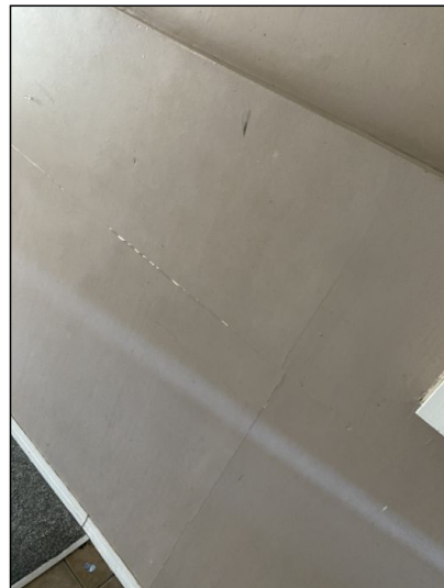
Some damaged walls noted throughout the house.
