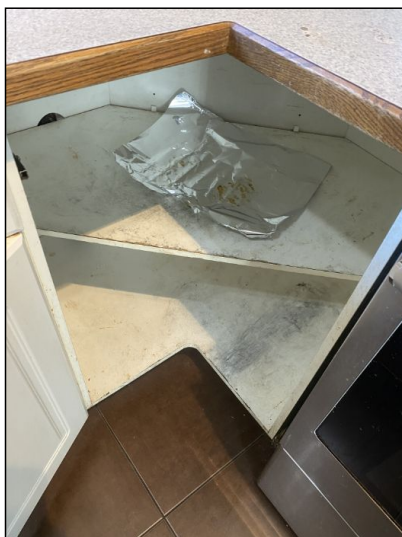
Cabinet door is missing.
