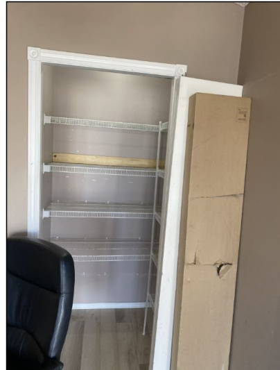
The closet door has fallen out of square or derailed and drags on the floor. We recommend contacting a qualified contractor to realign the door.
