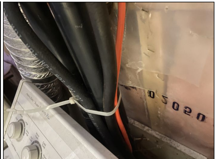
Operational/Functional at the time of inspection. No deficiencies observed.
