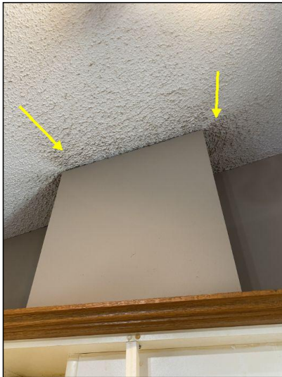
Appears to be leaking inside by the sealing recommend repair by qualified contractor.
