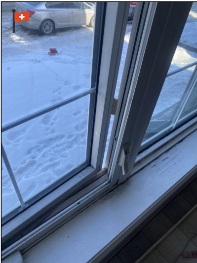
Front window did not lock/latch properly, recommend repairs for enhanced security/safety.
