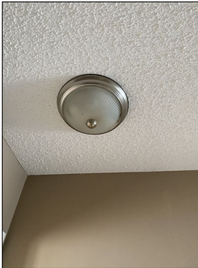
Non-functional light noted.
