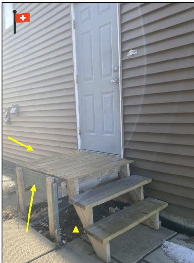
Handrail should be installed for safety.
