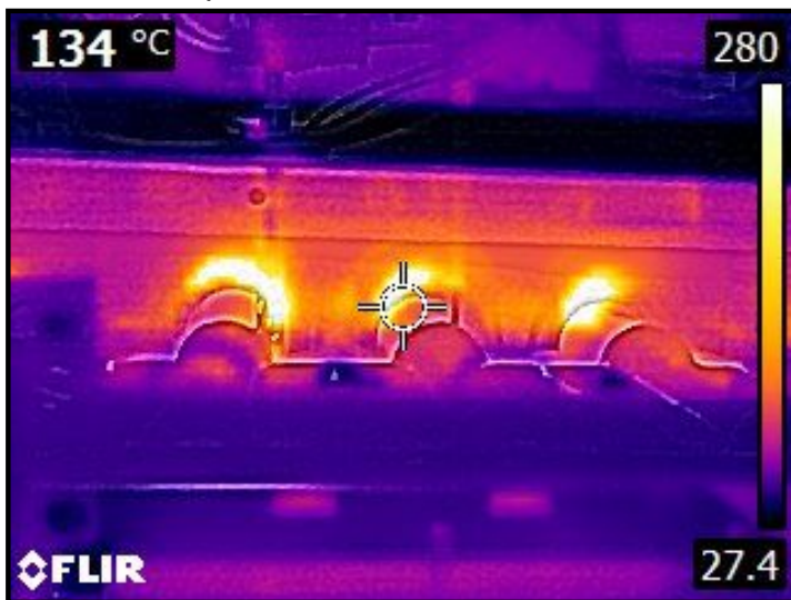
Gas fired forced hot air heating furnace was functional and operational at the time of inspection. Location: Basement.
