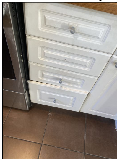
Cabinet door is missing and few other cabinet doors observed damaged.
