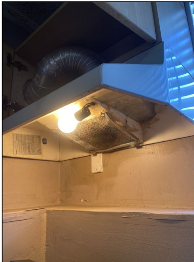
Exhaust fan was operational at the time of inspection. Tested suction.
