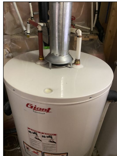
The water heater enclosure is functional.
