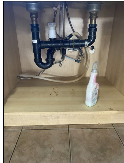
Operational/Functional at the time of inspection. No deficiencies observed.
