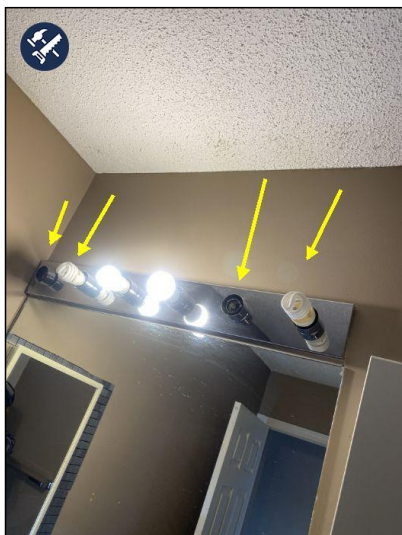
Light bulbs are missing at various locations recommend installing new bulbs or repair as necessary by qualified electrician.
