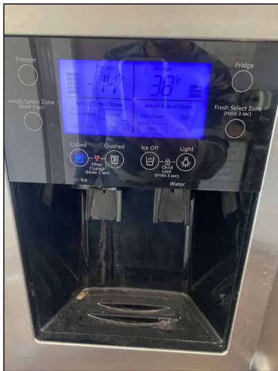
Water and ice dispenser is inoperable and the door handle observed missing.
