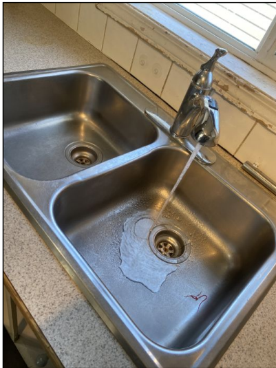
Operated normally, at time of inspection.
