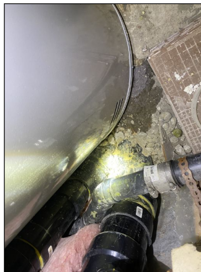
Main shut off valve located in the basement and the valve handle observed slow leaking. Recommend repair by qualified plumber.
