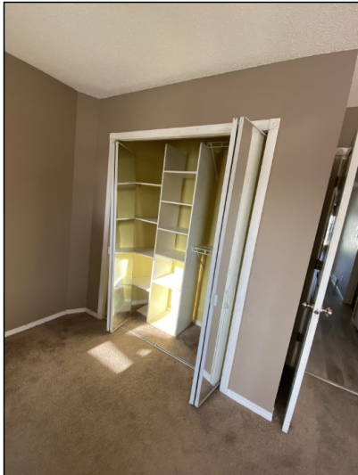
The closet door has fallen out of square or derailed and drags on the floor. We recommend contacting a qualified contractor to realign the door.
