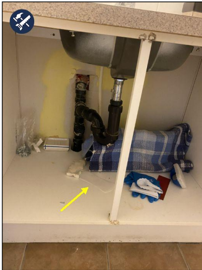
Visible leaking noted under the sink. We recommend contacting a licensed plumbing contractor for repair options.
