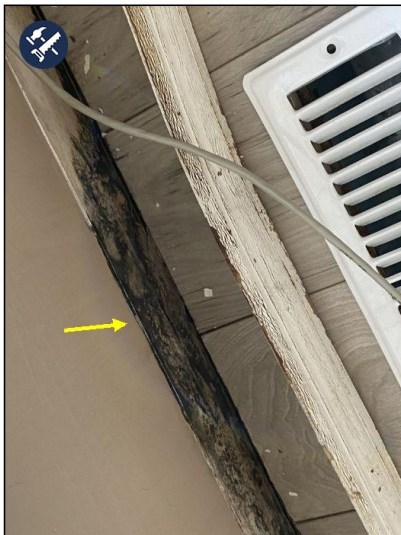
Mold like stains are present under the baseboard. We recommend further evaluation by qualified contractor.
