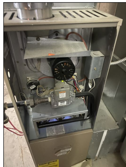
Gas fired forced hot air heating furnace was functional and operational at the time of inspection. Location: Basement.
