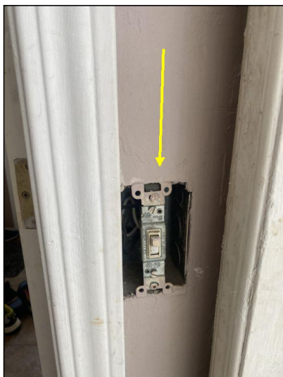
Missing outlet and switch covers Recommend installing new covers.
