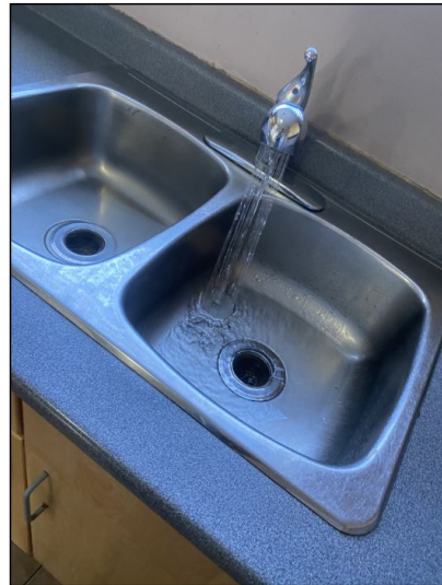
Operated normally, at time of inspection.
