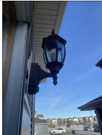
Front door outside light non-functional noted. Recommend repair by qualified electrician or replace bulb.
