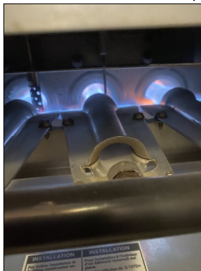
Gas fired forced hot air heating furnace was functional and operational at the time of inspection. Location: Basement.
