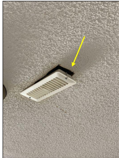
Recommend securing vent cover to sealing.
