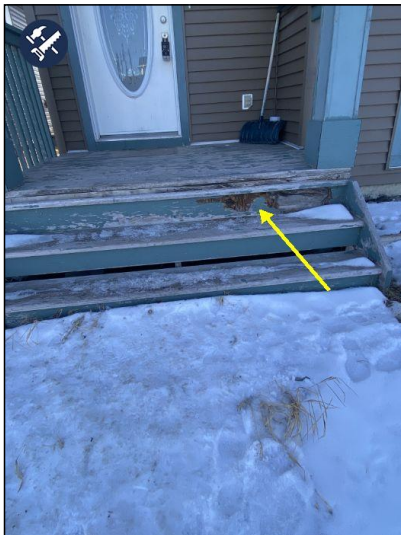
Front and side deck Floor boards rotted. Recommend repair by qualified contractor.
