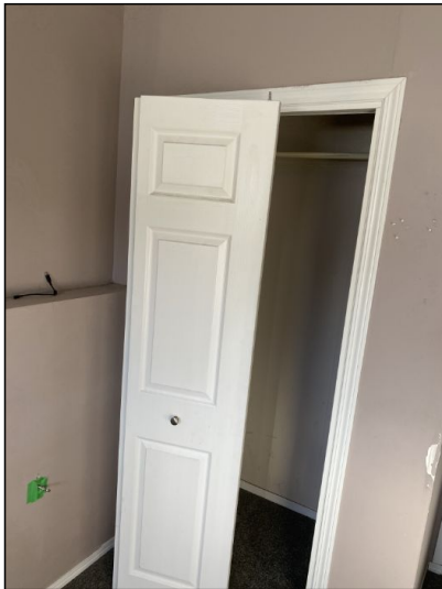
The closet door has fallen out of square or derailed and drags on the floor. We recommend contacting a qualified contractor to realign the door.
