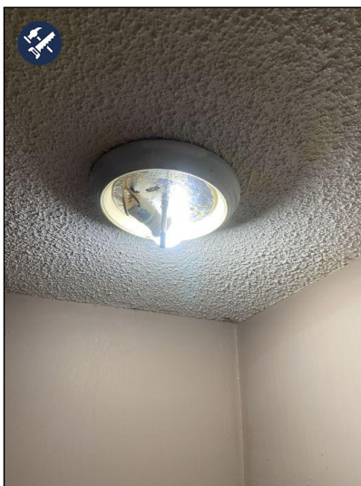
Light bulbs are missing at various locations recommend installing new bulbs or repair as necessary by qualified electrician. Recommend installing a cover on this light.
