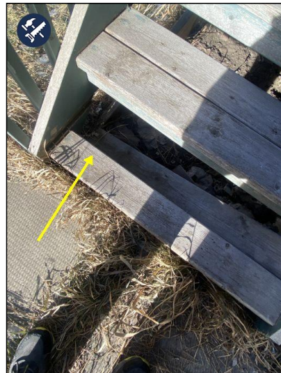
Front and side deck Floor boards rotted. Recommend repair by qualified contractor.
