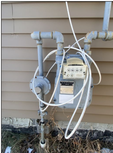
Meter located at exterior. All gas appliances have cut-off valves in line at each unit. No gas odors detected.
