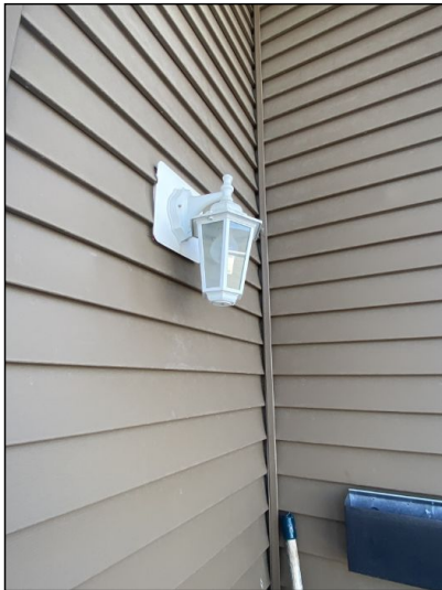
Front door outside light non-functional noted. Recommend repair by qualified electrician or replace bulb.
