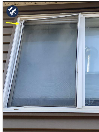
Some window screens damaged. And screen frame damage noted.
