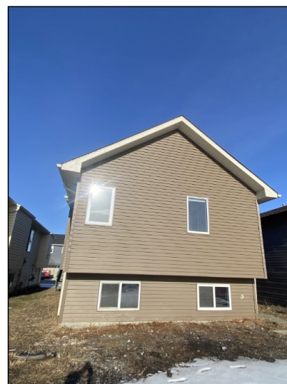
No major system safety or function concerns noted at time of inspection. Appeared functional at time of inspection. No deficiencies observed. Cosmetic damages are not included in the inspection report.
