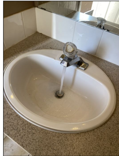
Operational/Functional at the time of inspection. No deficiencies observed. Cosmetic damages are not included in the inspection report.
